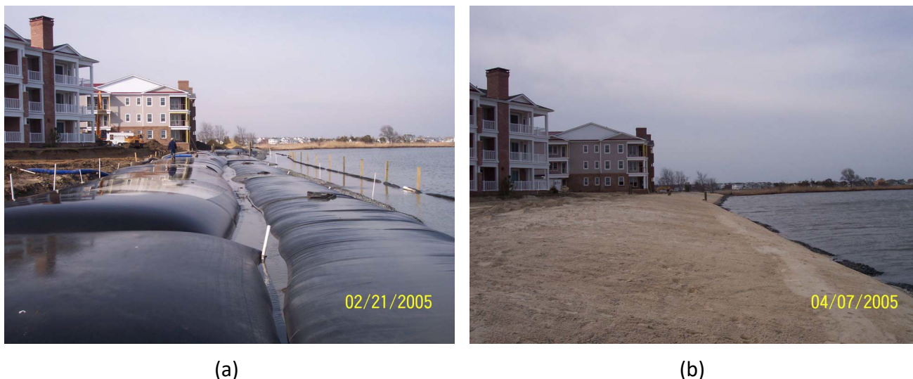
Figure 12. Photos. Shoreline stabilization with (a) geobags being filled and (b) finished revetment (De Gennaro, 2005).
