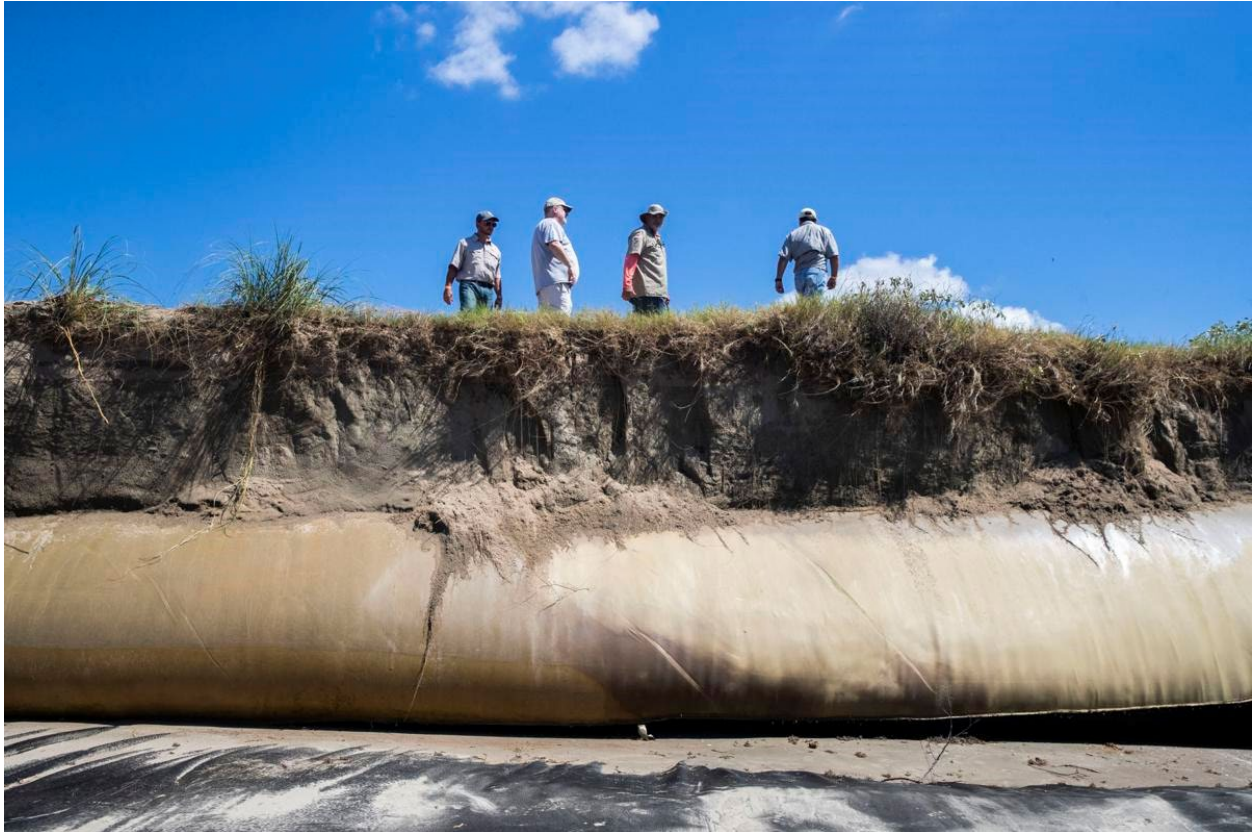
Figure 12. Photo. Officials inspect the damage to levees in Grand Isle, Louisiana, on Thursday, June 11, 2020 (Baurick, 2020).
