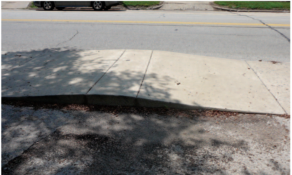
Driveway alignment taking precedent over sidewalk alignment does not meet accessibility requirements.
