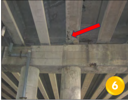
Two strands of reinforcement bars exposed in the bottom of beam
