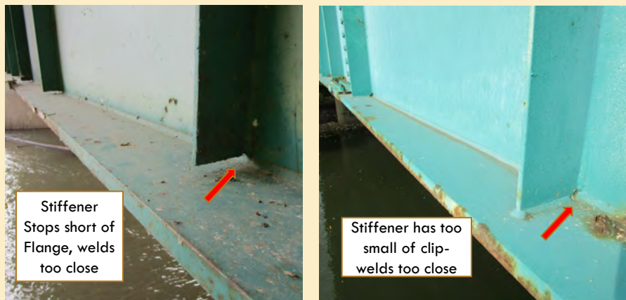
POOR Web Stiffener connection details – look at ends of plates in tension zones of girders
