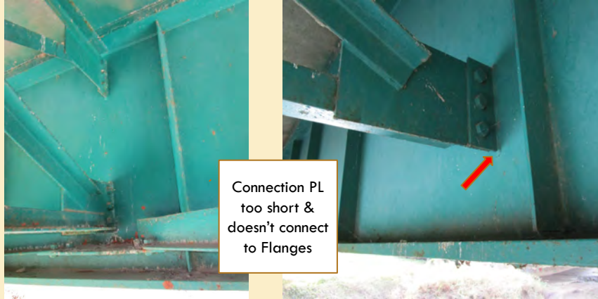
POOR Cross Frame connection details – look at ends of plates in tension zones of girders
